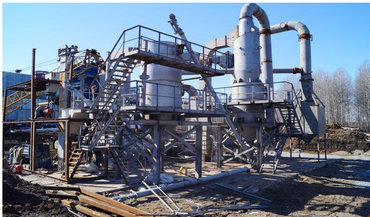
Figure 2. The picture of the equipment for milled brown coal heat-treatment and enrichment (testing bench) intended for the obtaining of carbon containing powders used in foundry. The equipment is undergoing the installation phase at the site of “Itatugol” LLC (Kemerovo region).
