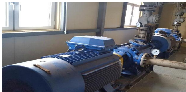
Fig.7. The injection electric pumps 180-340 of the centrifugal multistage sectional type for hot water with a gland seal installed in the pump station.
