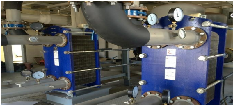
Fig.6. The plate heat exchangers "Ridan" installed in the GSCL heating unit.
