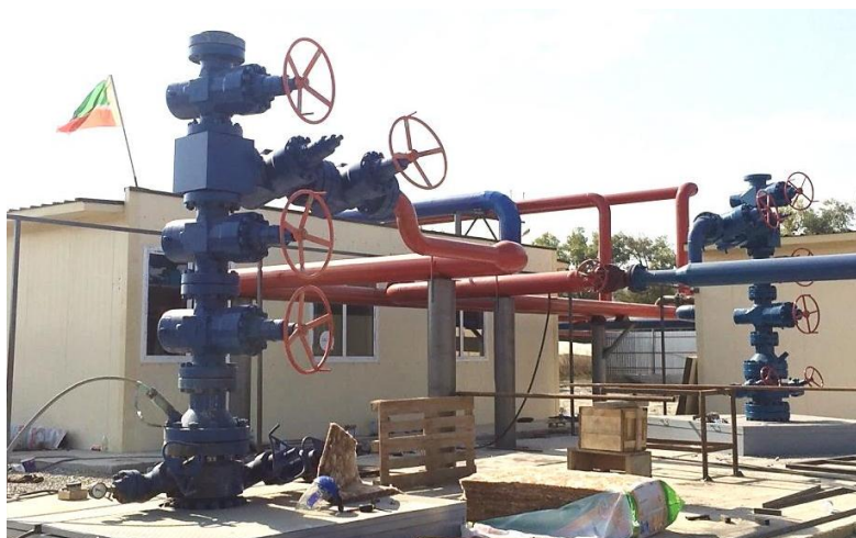
Fig.5. The water production and injection wellheads.
