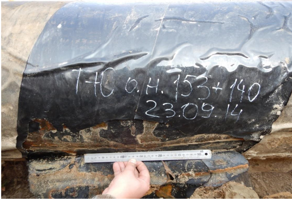
Figure 4: Check pit on the pipeline T-Yu made based on the results of the diagnostic test.
