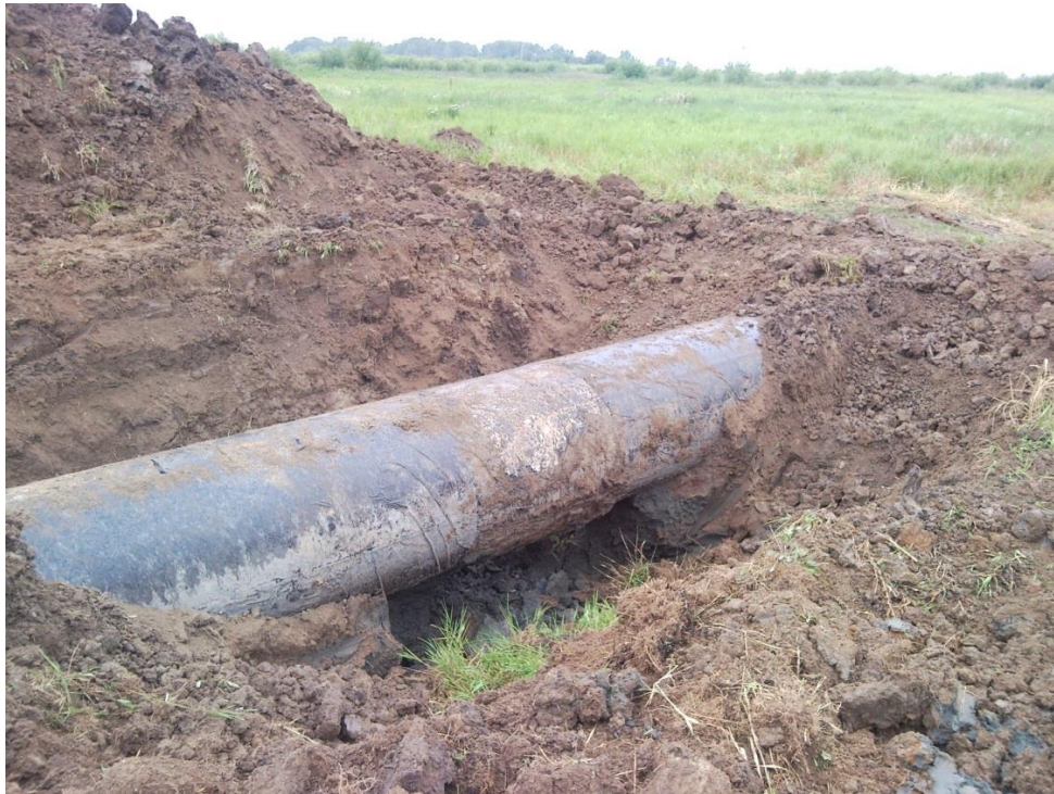
Figure 2: Check pit on the pipeline UBKUA made based on the results of the diagnostic test
