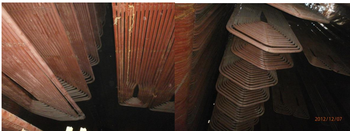
Figure 1: Inner view of the PF boiler (Super heater coils)
